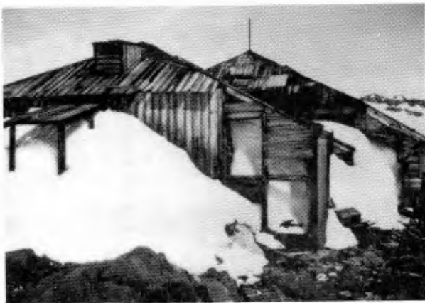
View of the hut showing snow accumulation in interior as at December 1981.
